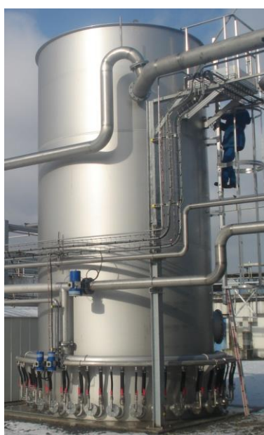
Figure 4. Biofiltration tank serving 3.000 Population Equivalents [photo: Aquabiotec]
